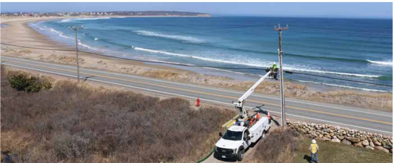
Winds were constantly monitored for safety in buckets extended 25 feet aloft. Block Island's strongest winds blew during prime construction months.
