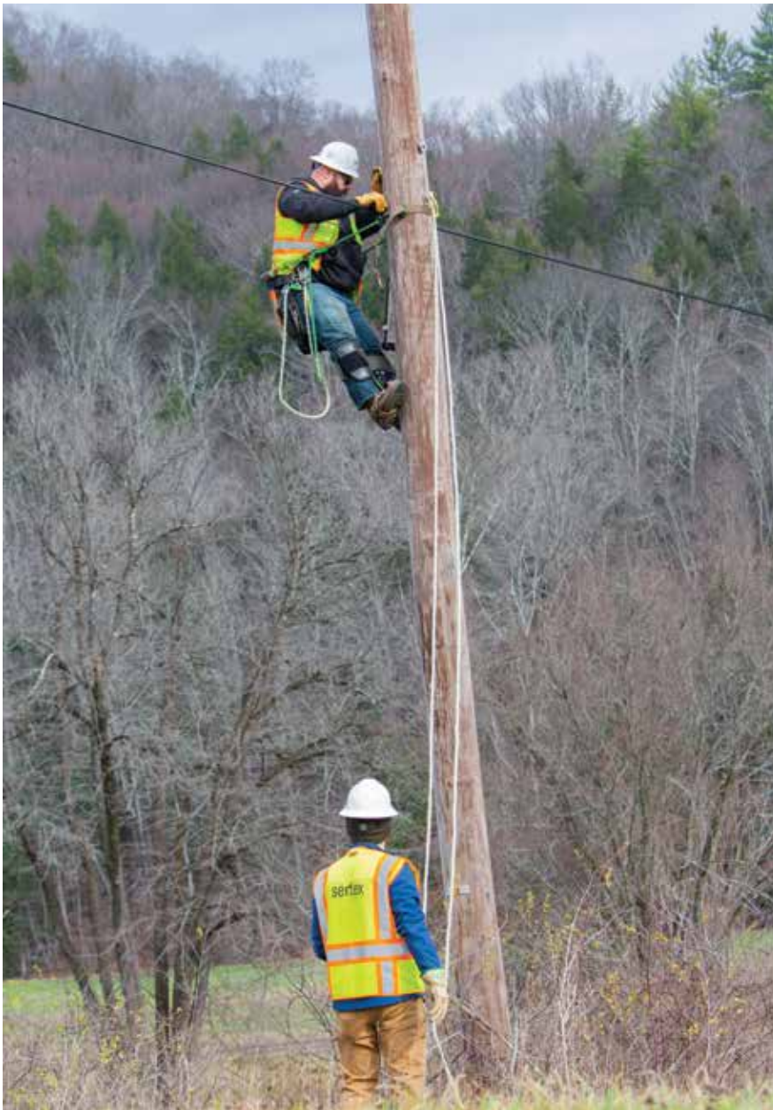
Once western Massachusetts utilities completed make ready and poles were licensed, Sertex crews were redirected to aerial cable installation.
