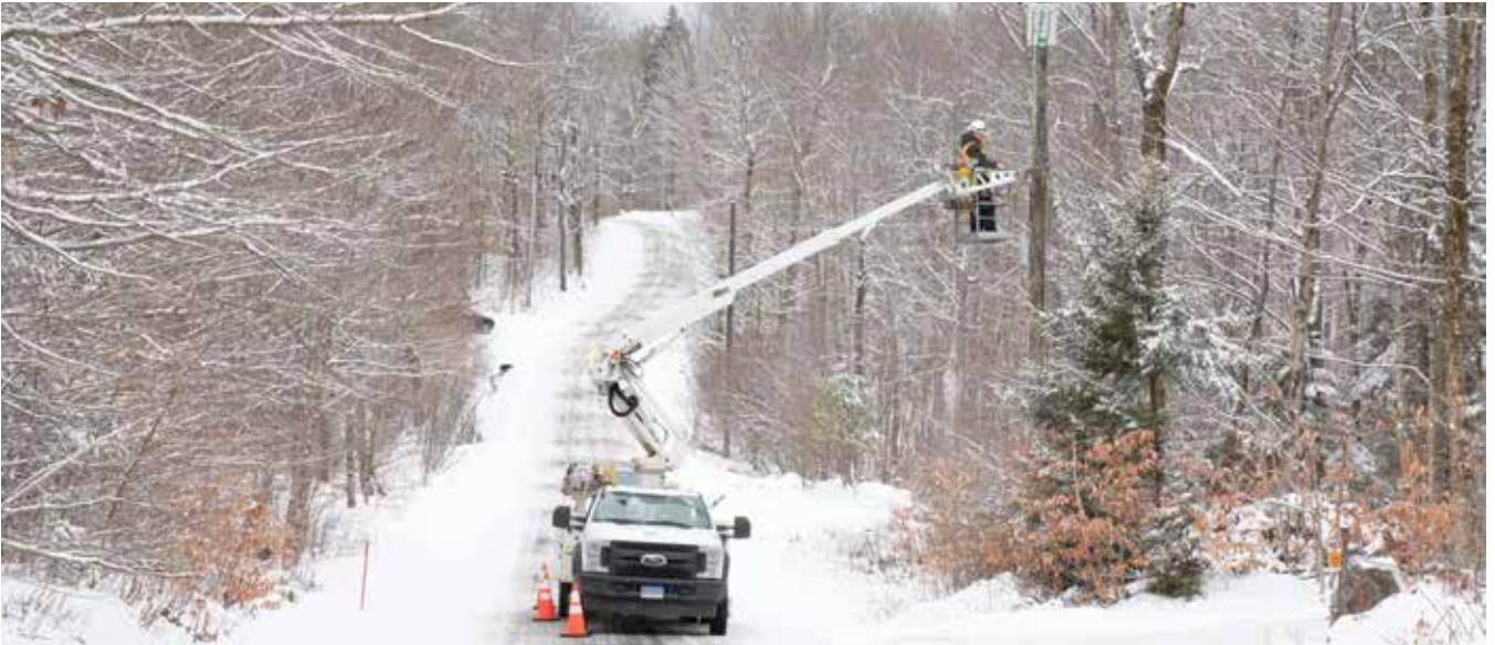
In high-elevation areas, the winter season lasts up to six months. Crews deploy fiber through challenging terrain and extreme weather conditions.
