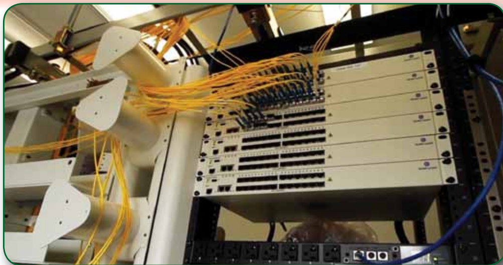
Equipment in a fiber aggregation hut.
