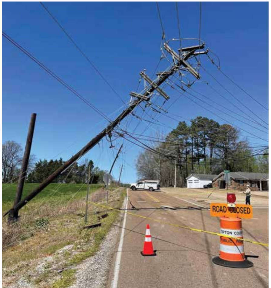
STEMC’s fiber crew finished the telecom restoration six hours after the electric repair.
